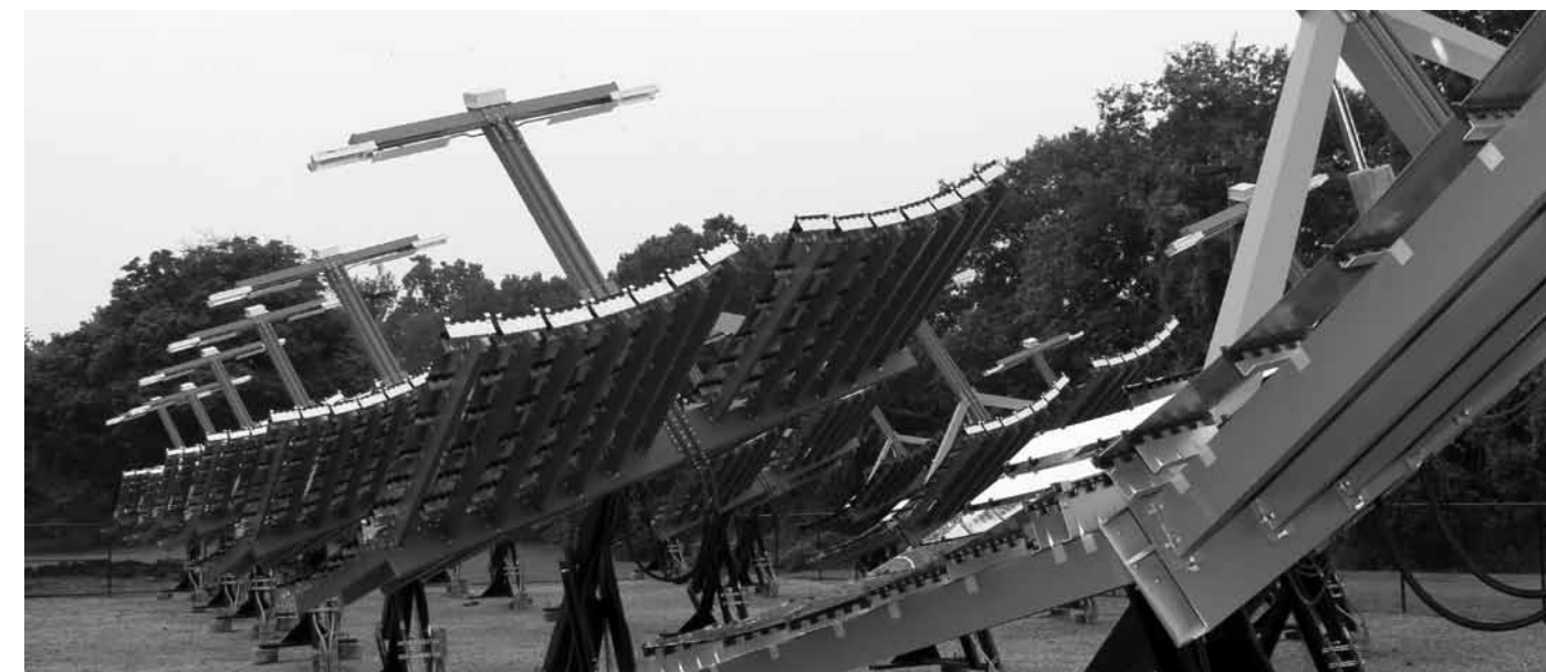
Twenty high-powered solar concentrators have been installed at Rockefeller Park greenhouse.
